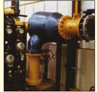
12" KSS Cyclone & Reservoir
